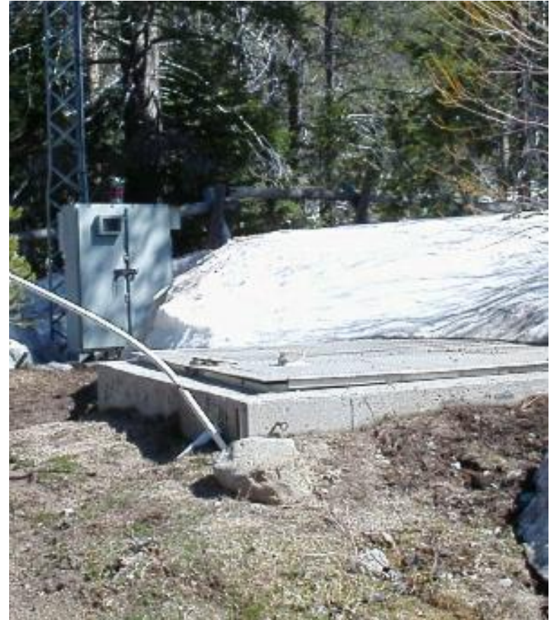
OVPD's East BPS & PRV vault
