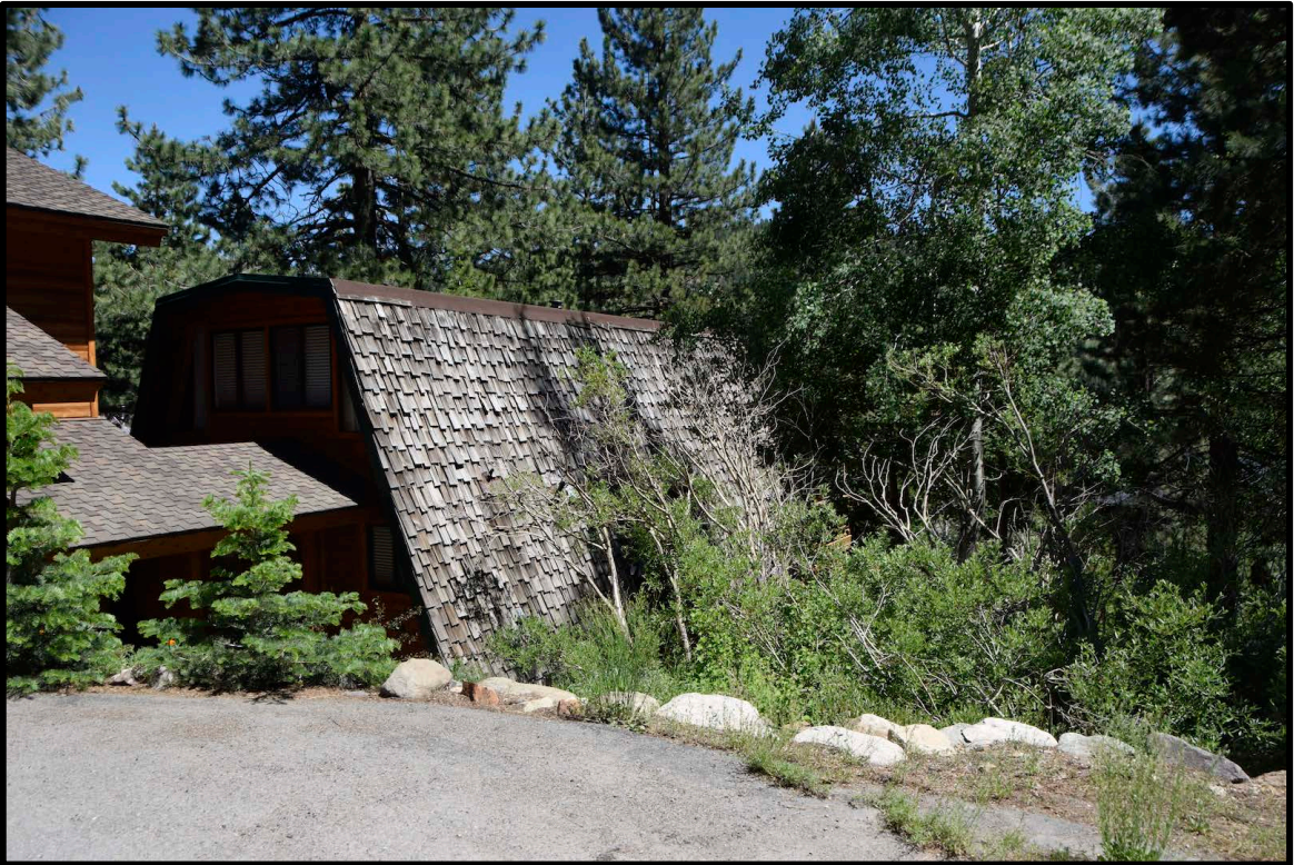
Figure 15: Dense vegetation growing right up against a wood-shingled house. Structure ignition hazard reduction techniques should be a major emphasis of education programs.
