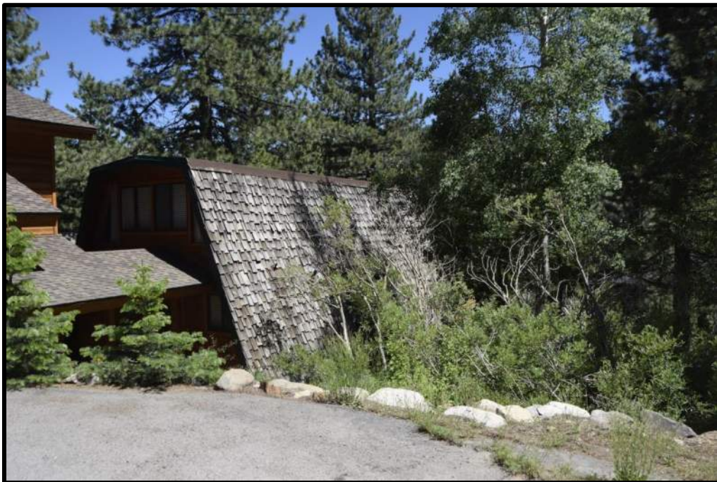
Figure 12: Dense vegetation growing right up against a wood-shingled house. Structure ignition hazard reduction techniques should be a major emphasis of education programs.
