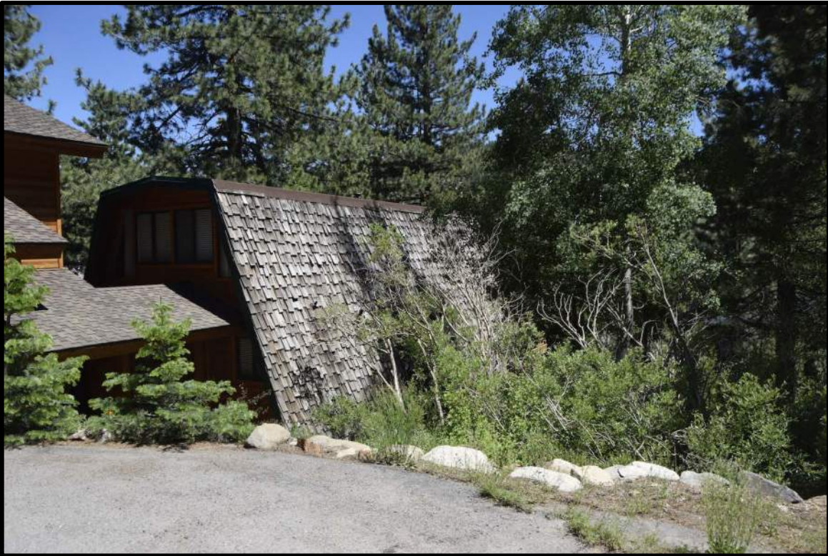
Figure 15: Dense vegetation growing right up against a wood-shingled house. Structure ignition hazard reduction techniques should be a major emphasis of education programs.
